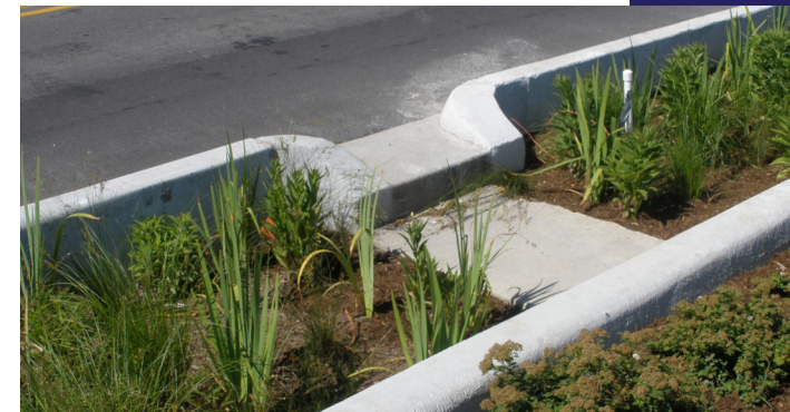
Bioswales treat runoff in Indianapolis
